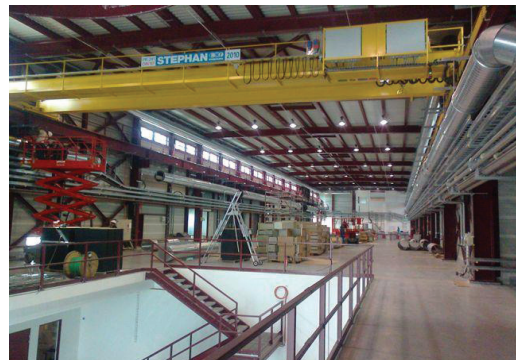
Figure 6: Linac4 equipment hall (May 2011).
