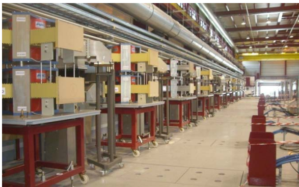
Figure 6: RF Network installed in the Linac4 Hall.
